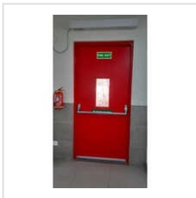
Metal Fire Doors
