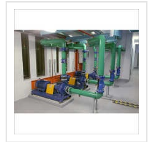
Chilled Water Systems
