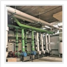
SITC Maintenance Of Chilled Water System
