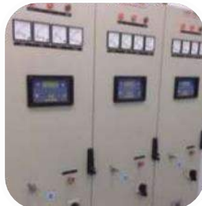
ESP CONTROL PANELS
