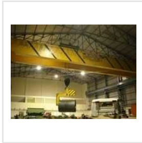
Double Girder Overhead Cranes
