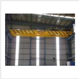
Double Girder Crane For Transformer
