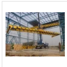
Industrial Eot Cranes
