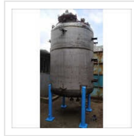
Mild Steel Storage Tank
