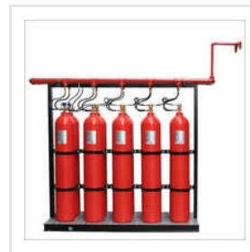
Co2 And FM200 Flooding Systems
