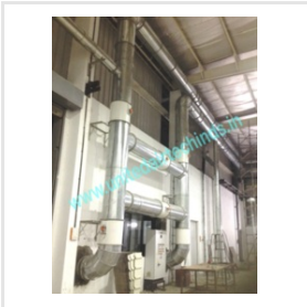
GI ROUND DUCTING
