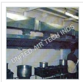
Kitchen Ventilation Systems
