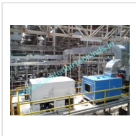
Industrial Fume Extraction System
