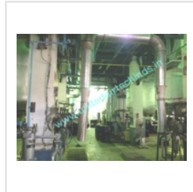
Industrial Air Ventilation System
