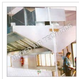
Kitchen Exhaust System
