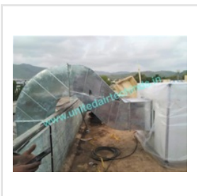
FRESH AIR VENTILATION DUCTING
