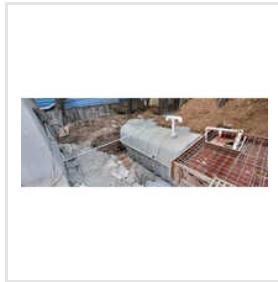
Residential Sewage Treatment Plant
