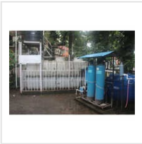
Johkasou Sewage Treatment FRP Plant
