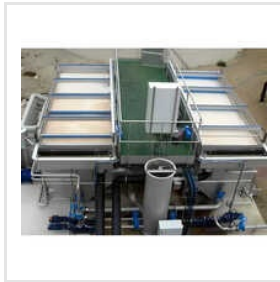
Commercial Water Treatment Plant
