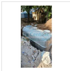
Sewage Treatment Plant At Sarswati
