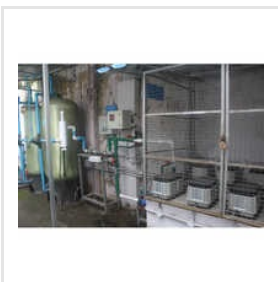
Industrial Sewage Treatment Plant
