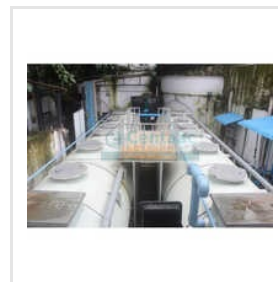
Compact Sewage Treatment Plant
