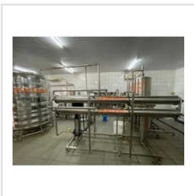
Packaged Water Treatment Plants
