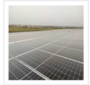
Industrial Solar Power System
