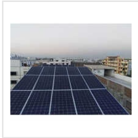
3.35KW Solar Power System
