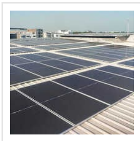
Solar Energy Power System
