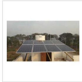
10.5KW Solar Power System
