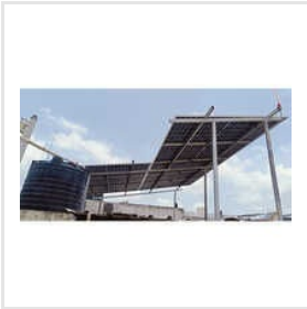
Industrial Solar Rooftop System
