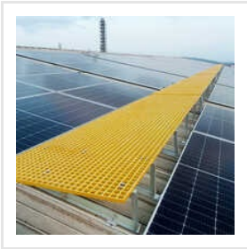
Solar Power Roof System
