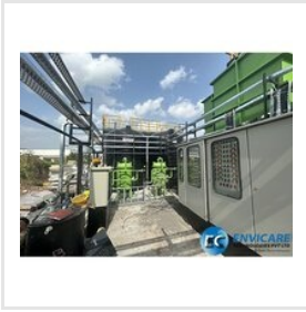
Effluent Treatment Plant
