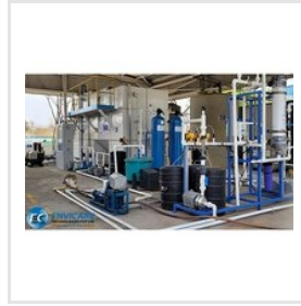
Sewage Treatment Plant With UF
