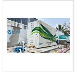
Containerised Sewage Treatment Plant
