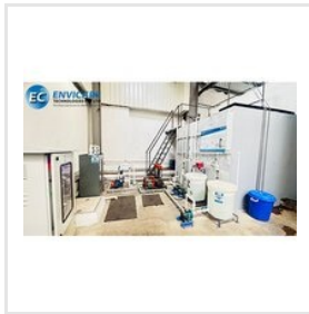
MBR Sewage Treatment Plant
