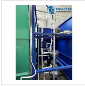
ZLD Effluent Treatment Plant
