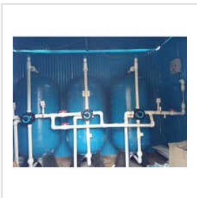
Industrial Fluoride Removal Plant
