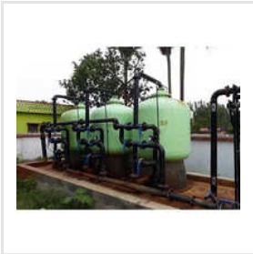
Arsenic Removal Plant
