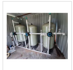
Domestic Iron Removal Plant
