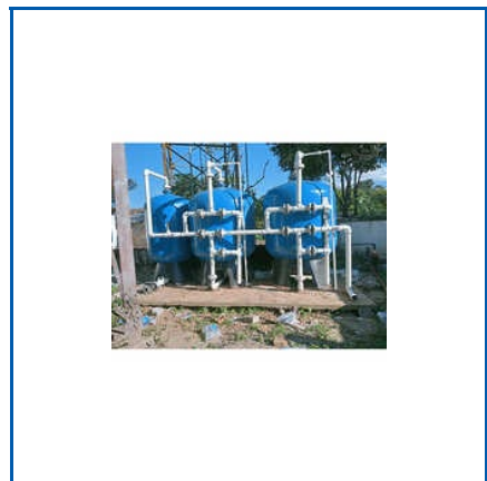
INDUSTRIAL IRON REMOVAL PLANT
