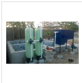
Industrial Sewage Treatment Plant
