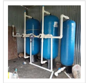
1000LPH Iron Removal Plant
