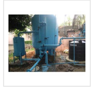
FRP Water Treatment Plant
