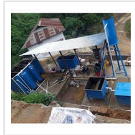
Industrial Effluent Treatment Plant
