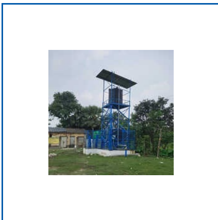
SOLAR BASED CPP UNIT
