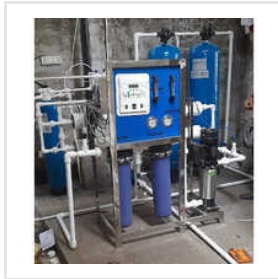
FRP Reverse Osmosis Plant
