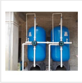
Industrial Water Treatment Plant
