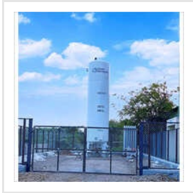
Liquid Oxygen Tank
