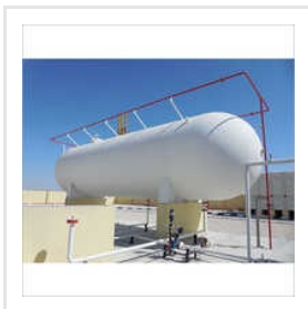
LPG Storage Tank
