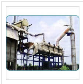
Waste Heat Thermic Fluid Heaters
