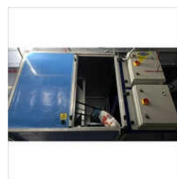
Dry Scrubber Unit
