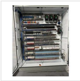
Industrial Control Panels
