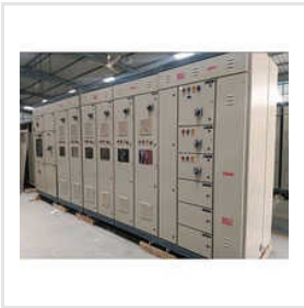
Industrial Power Panels
