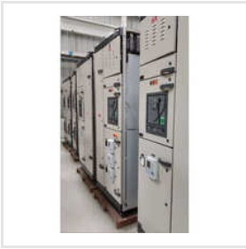
PCC Control Panel
