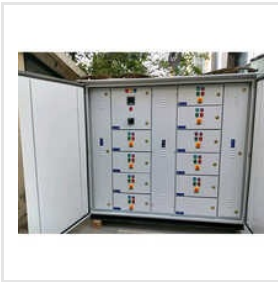
Motor Control Panel
