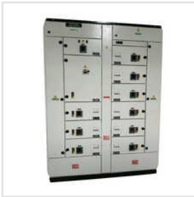
Critical UPS Outgoing Panel
