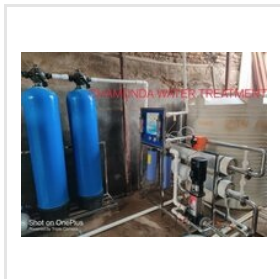
2000 LPH FRP Industrial RO Plant
