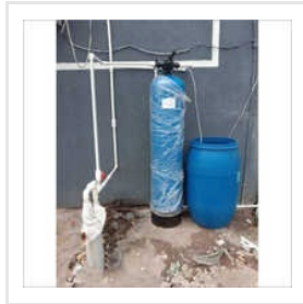
Pentair Water Softener Plant
