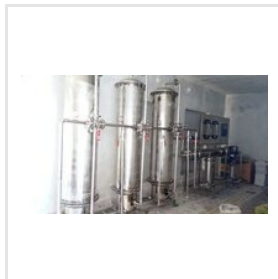
Drinking Water Plant
