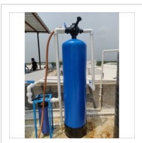
RO Water Softener Plant
