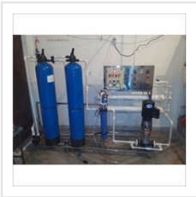
Industrial Reverse Osmosis Plant
