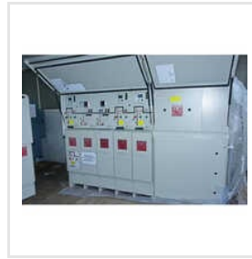
Siemens 11 KV Ring Main Unit
