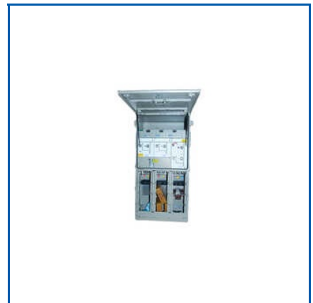
INDUSTRIAL RING MAIN UNIT
