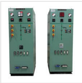
Control And Relay Panel
