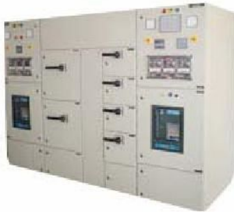
POWER DIST. BOARD
