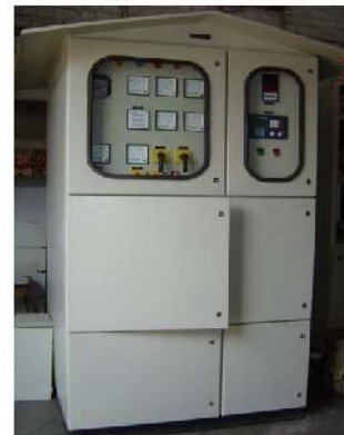
D.G. CONTROL PANEL
