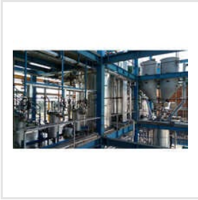
Palm Oil Refinery Plants
