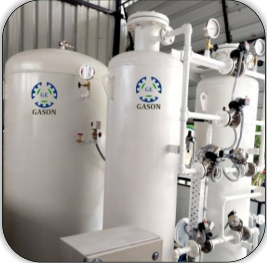
Medical PSA Oxygen Gas Plant
