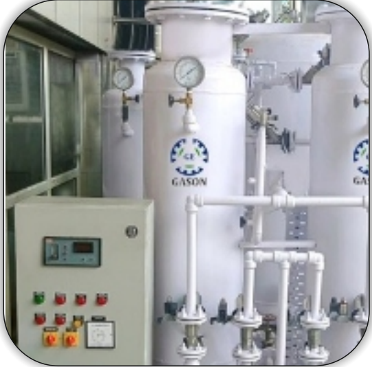
PSA Nitrogen Gas Plant
