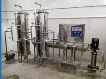
SS RO Plant
