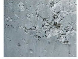
Cracks - Honeycombs Services
