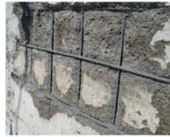
Spalling Of Concrete Services
