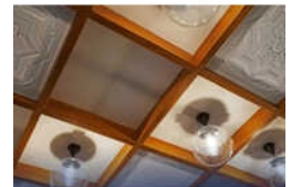
Grid False Ceiling
