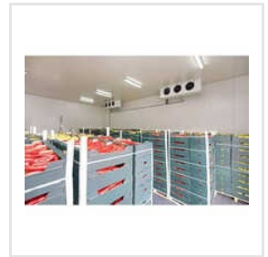
Commercial Cold Storage Room
