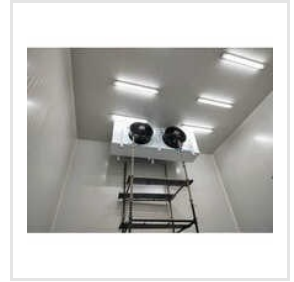
Blue Star Cold Storage Room
