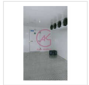
Cold Storage Room
