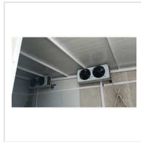
Commercial Cold Room
