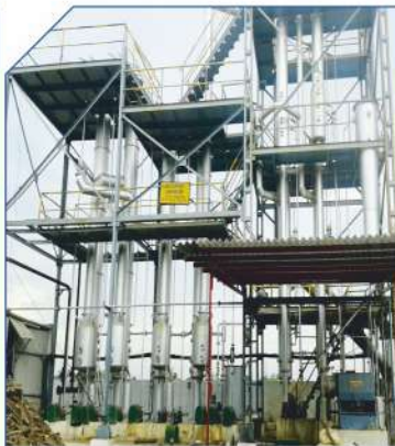
ANGERIPALAYAM CETP PVT LTD - 200 KLD
