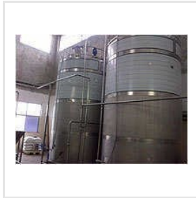
Stainless Steel Tank
