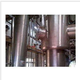
Large Scale Evaporators
