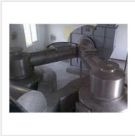
Industrial Spray Dryer
