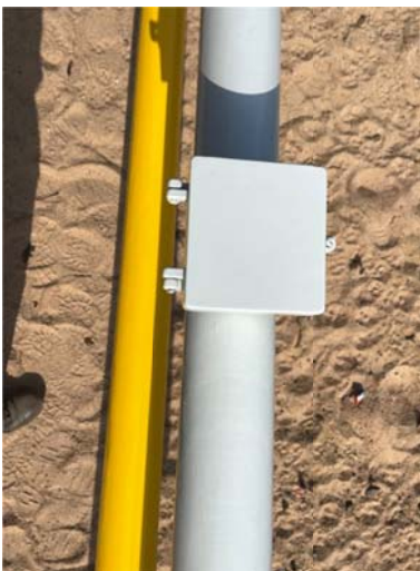
External junction box
