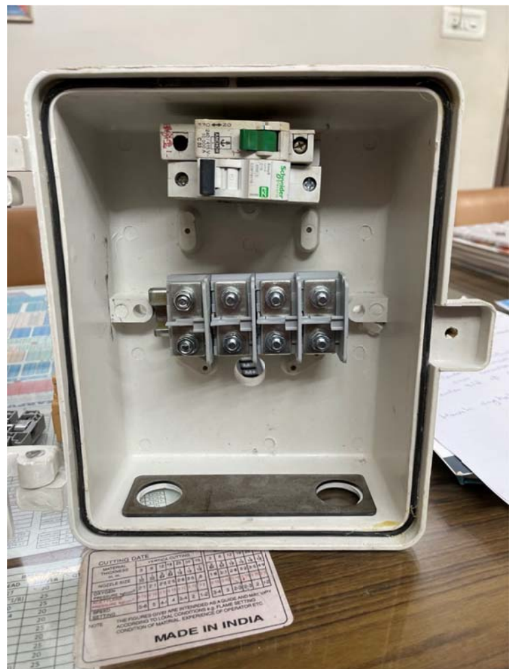
External junction box with connectors & MCB
