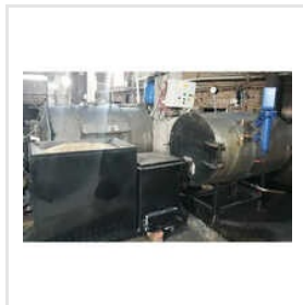
Pellet Fired Steam Boiler
