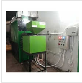
Gas Fired Hot Air Generator
