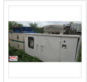
Used Diesel Generator
