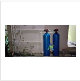
500 LPH Iron Removal Plant
