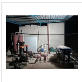
1000 KLD Sewage Treatment Plant
