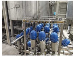
Industrial Valve Cluster
