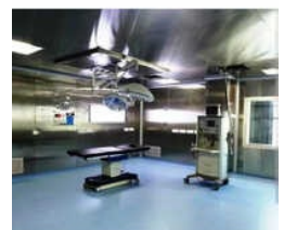
Hospital Operation Theater
