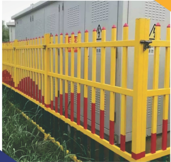
FRP TRANSFORMER FENCING
