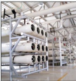
Industrial Ro. Plant
