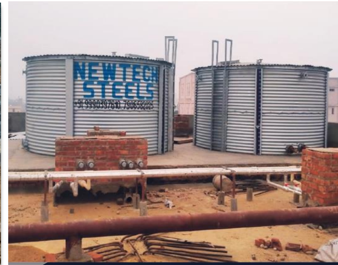
Overhead tanks (on the roof)
