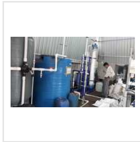
Industrial Ultrafiltration Plant
