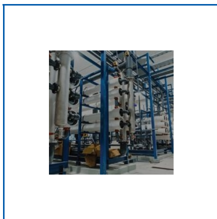
REVERSE OSMOSIS PLANT – RO PLANT
