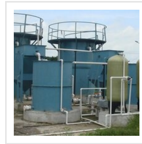
Effluent Treatment Plant ETP
