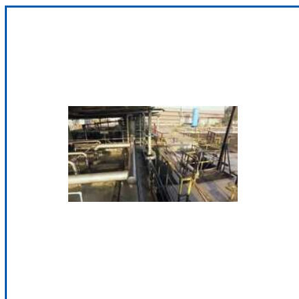
ZERO LIQUID DISCHARGE SYSTEM
