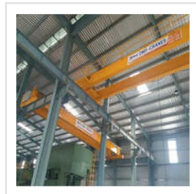
Double Girder Bridge Crane
