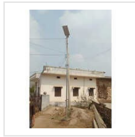
18 Watt Solar Inbuilt Street Light
