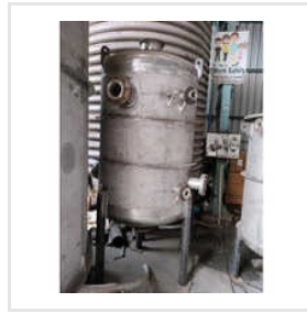
Stainless Steel Water Storage Tank
