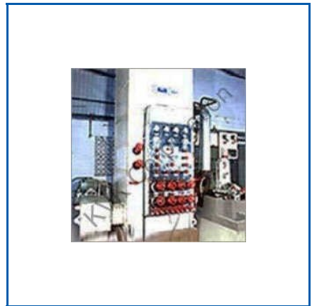
INDUSTRIAL OXYGEN GAS PLANT
