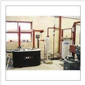
Industrial Nitrogen Gas Plant
