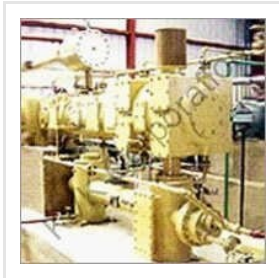
KVK Nitrogen Gas Plant
