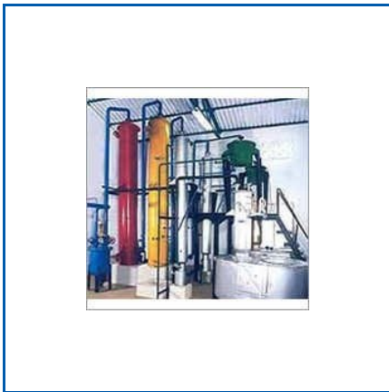
INDUSTRIAL NITROUS OXIDE PLANT
