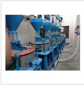
Flour Mill Plant
