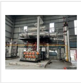
Co2 Liquefaction Plant
