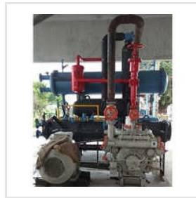
Industrial Ammonia Refrigeration System
