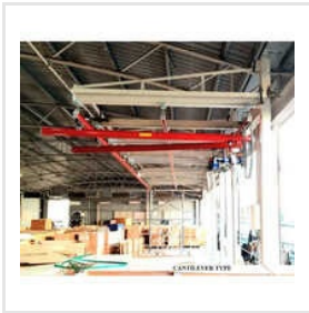
Galvanized Steel KBK Rail System
