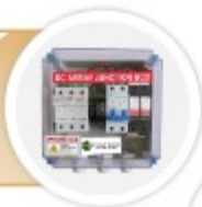
PV Combiner Box
