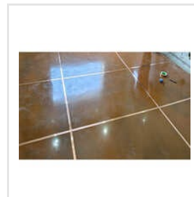
Electrostatic Discharge Flooring
