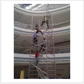
Aluminium Scaffold Tower
