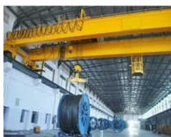
Double Beam EOT Crane
