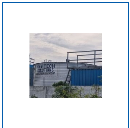
INDUSTRIAL WATER STORAGE TANK
