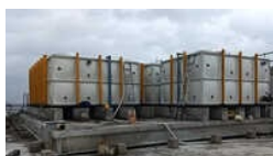
Grp Panel Water Tank
