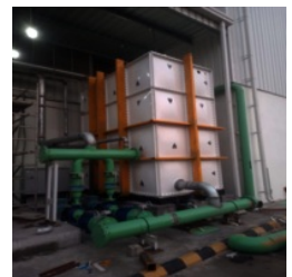
Fire Grp Water Storage Tanks
